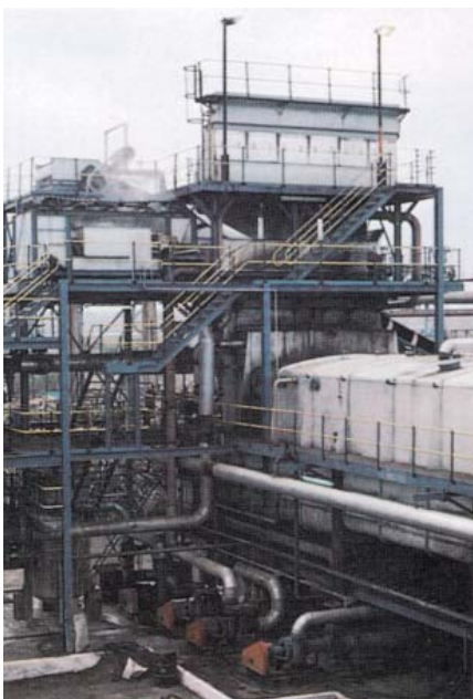
View of cane diffuser inlet
